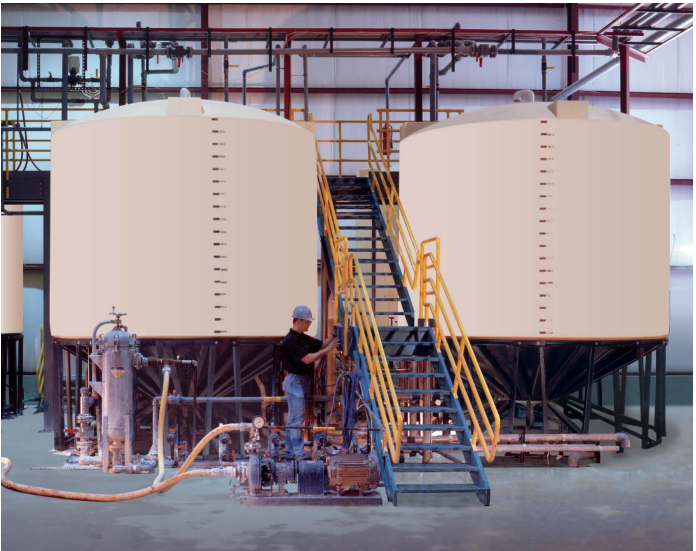
Assmann conical bottom storage tanks at a central Indiana chemical company.
